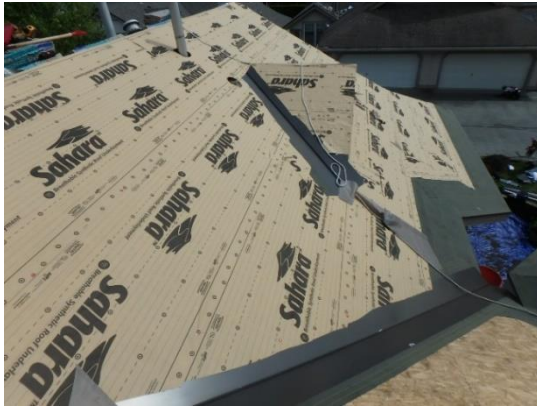
View of new underlayment, flashings, and accessories being installed at a sloped roof prior to asphalt shingle installations.
