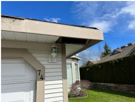
View of fascia board replacement work in progress prior to installing the new gutters and downpipes.
