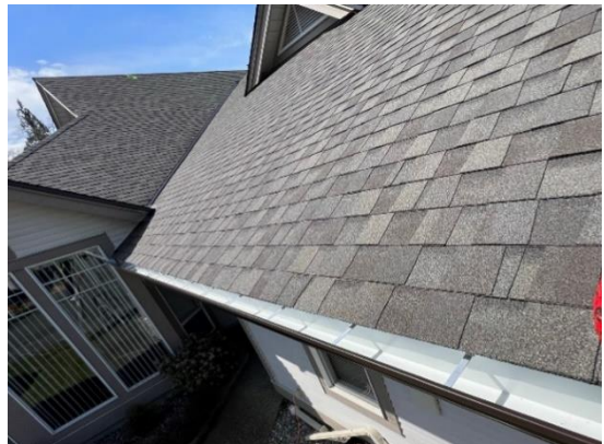
View of new aluminum gutter in place along a sloped roof eave.
