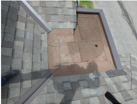
View of new 2-ply SBS modified bitumen sheet membrane assembly at a flat roof.
