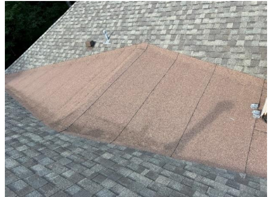
View of new 2-ply SBS modified bitumen sheet membrane assembly at a low-slope roof.
